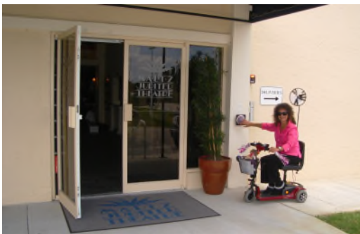
Susan Arena @ Maltz Theatre after installation of Horton Automatic Opener.
